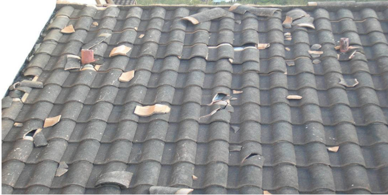
Photo 1: Mortar set roof system, with wind damage over 25%.
