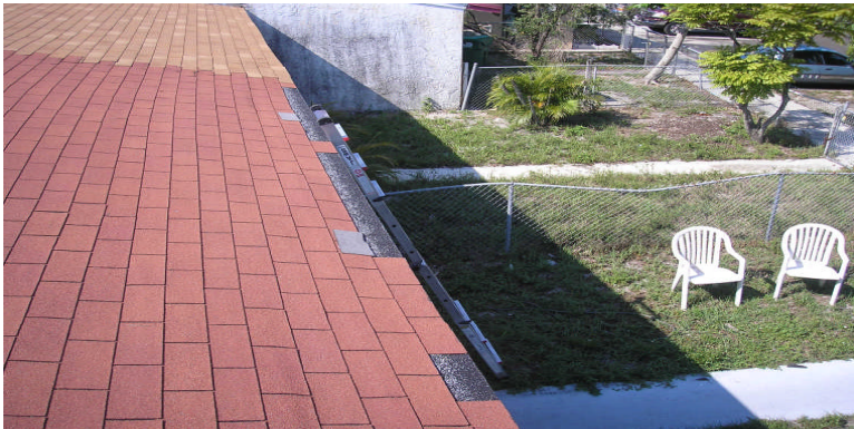
Photo 7: Asphalt shingle roofing with minimal wind damage.
