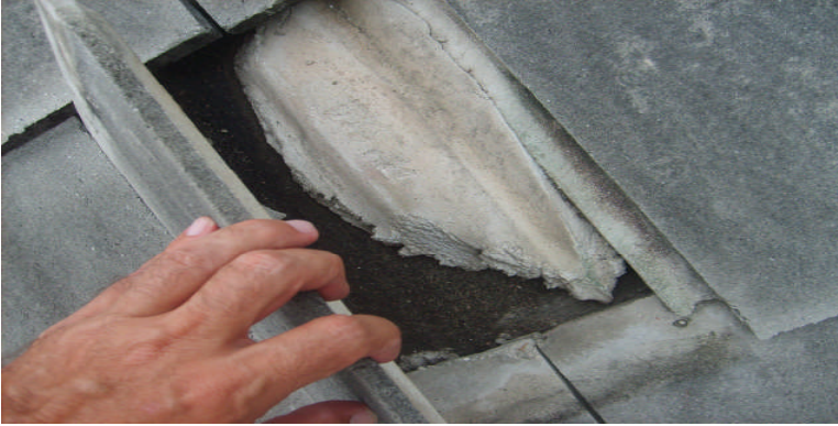
Photo 3: Loose tiles in place with the failure plane between the tiles and the mortar.
