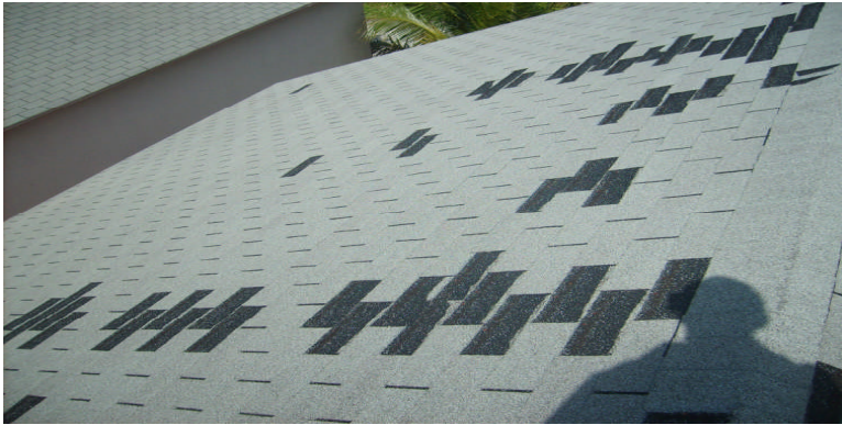
Photo 6: Asphalt shingle roofing with wind damage over 25% to the entire roof area.
