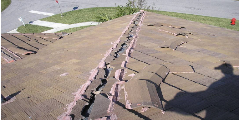
Photo 5: Nail down roof tiles with minimal wind damage to the field tiles.
