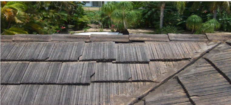
Photo 4: Nail down roof tiles with wind damage to the field tiles.
