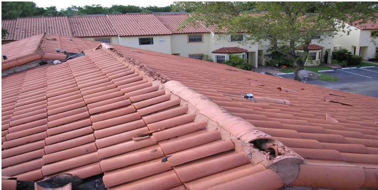
Photo 2: Foam set roof system with scattered roof ridge tiles and minimal wind damage to the field tiles. (Ridge tiles installed with mortar only.)
