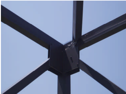
Figure 7 – Distress at connections
