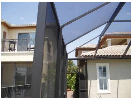
Figure 4 – Leaning of screen walls
