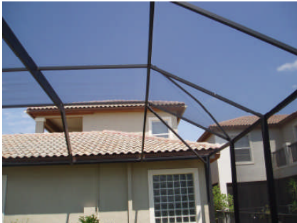
Figure 6 – Failure of diagonal braces
