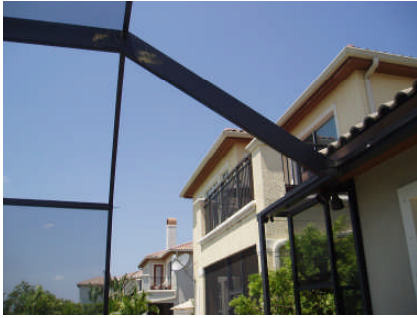
Figure 5 – Missing diagonal members and screens
